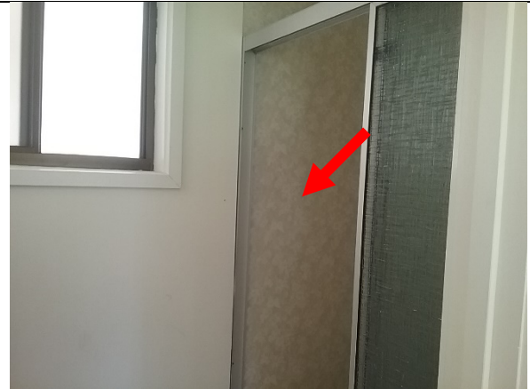
Photo 9: Tilux surfaces of shower in Laundry/Toilet visually identified as asbestos.
