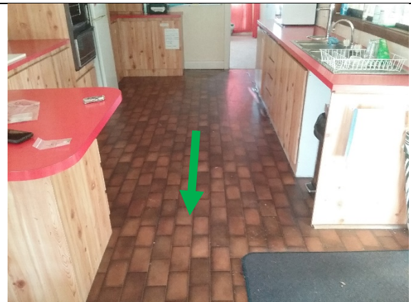
Photo 5: No asbestos detected in sample 4-270721. Vinyl sheet on timber floor of Kitchen/Dining.
