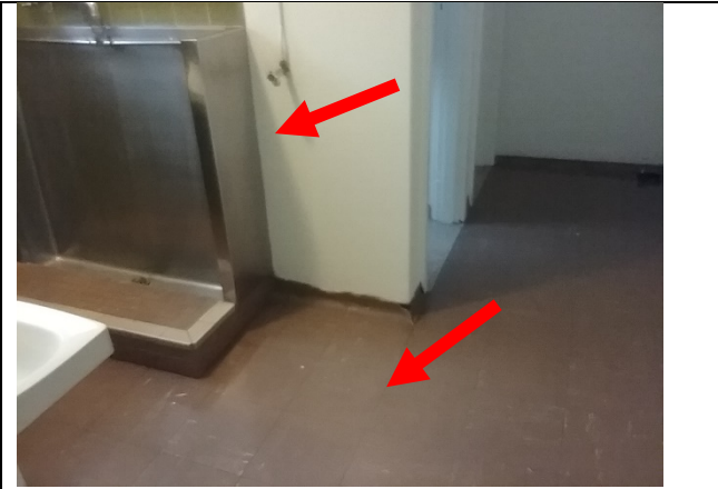
Photo 2: Asbestos detected in representative sample 1-230721. Vinyl tile floor in male toilet. Possible cement sheet behind urinal. Assume asbestos is present until determined otherwise.
