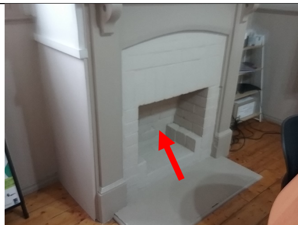
Photo 4: No access inside hallway and dining room fireplace at the time of the audit. Assume asbestos is present until determined otherwise.
