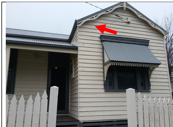
Photo 1: No access to eaves due to fall hazard. Assume asbestos is present until determined otherwise.
