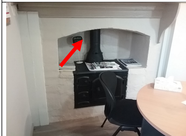
Photo 5: No access inside kitchen fireplace at the time of the audit. Assume asbestos is present until determined otherwise.
