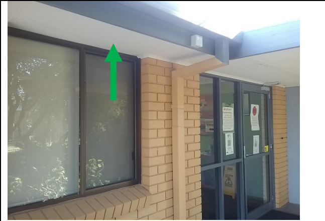
Photo 2: No asbestos detected in sample 1-270721. Cement sheet eaves of Main building.
