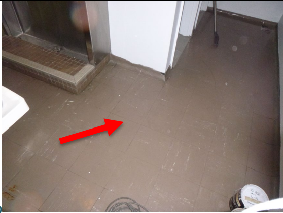
D Photo 349: Asbestos detected in sample 01-230721. Vinyl tile floor in staff toilet.
